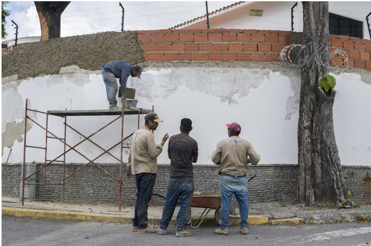
Figure 3. Construction of additional layers on existing perimeter wall. Photo by Edgar Martínez
