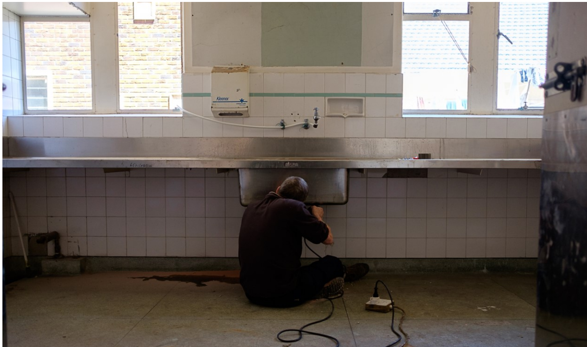
Figure 2. Uncle Freddy fixes a leak in a sink after connecting a water pipe
