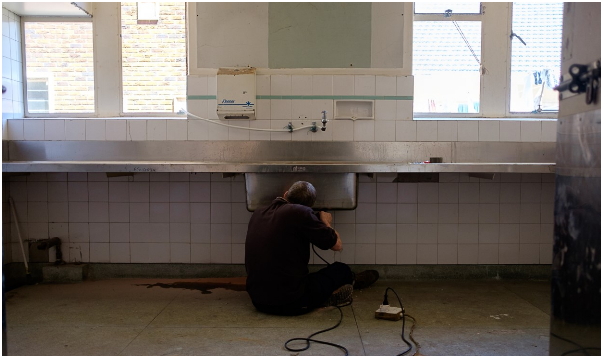
Figure 2. Uncle Freddy fixes a leak in a sink after connecting a water pipe
