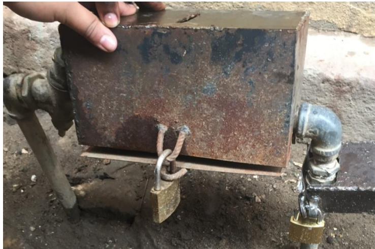
Figure 1. Steel case and pad-lock to control water availability to tap-users. Source: Author's original
